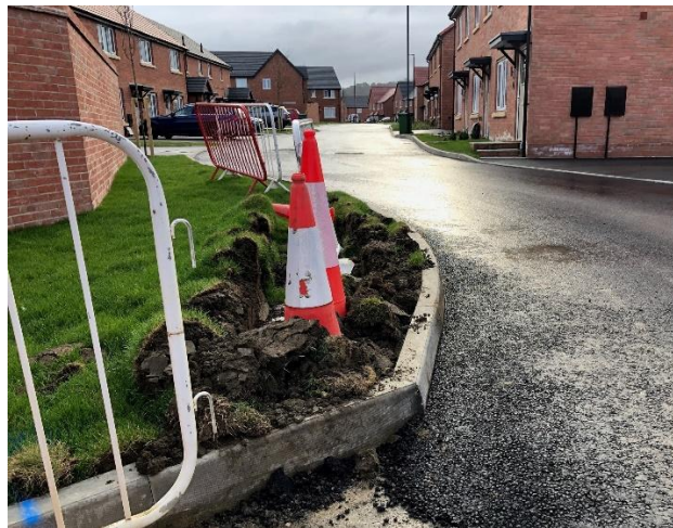
Poorly designed roads lead to verge damage
